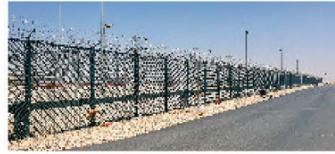
New Sudair 380kv substation, KSA
