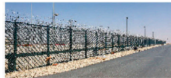
New Sudair 380kv substation, KSA
