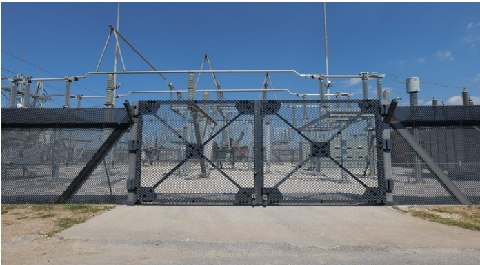
Double swing vehicle gate on a switchyard entry, braced and non-conductive through the leaf.
