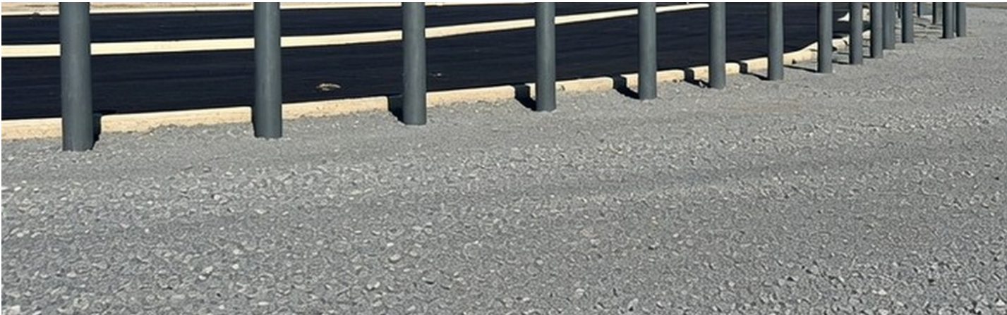
Crash-rated bollard run at a federal facility, set flush with the drive surface.
