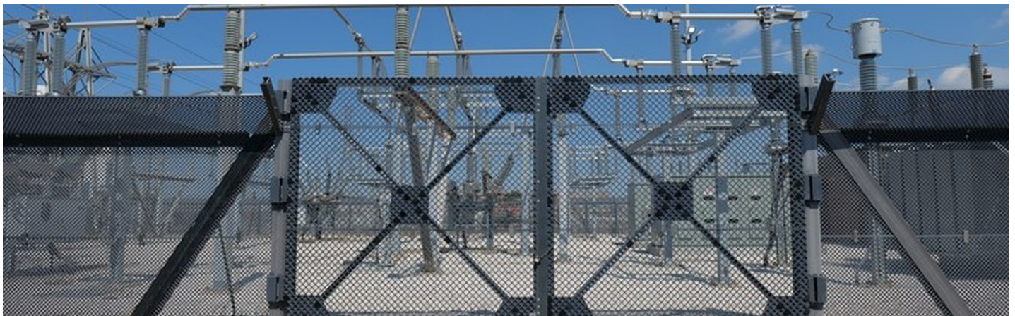
ENC fence and gate at an energized substation. No conductive path, no additional grounding.
